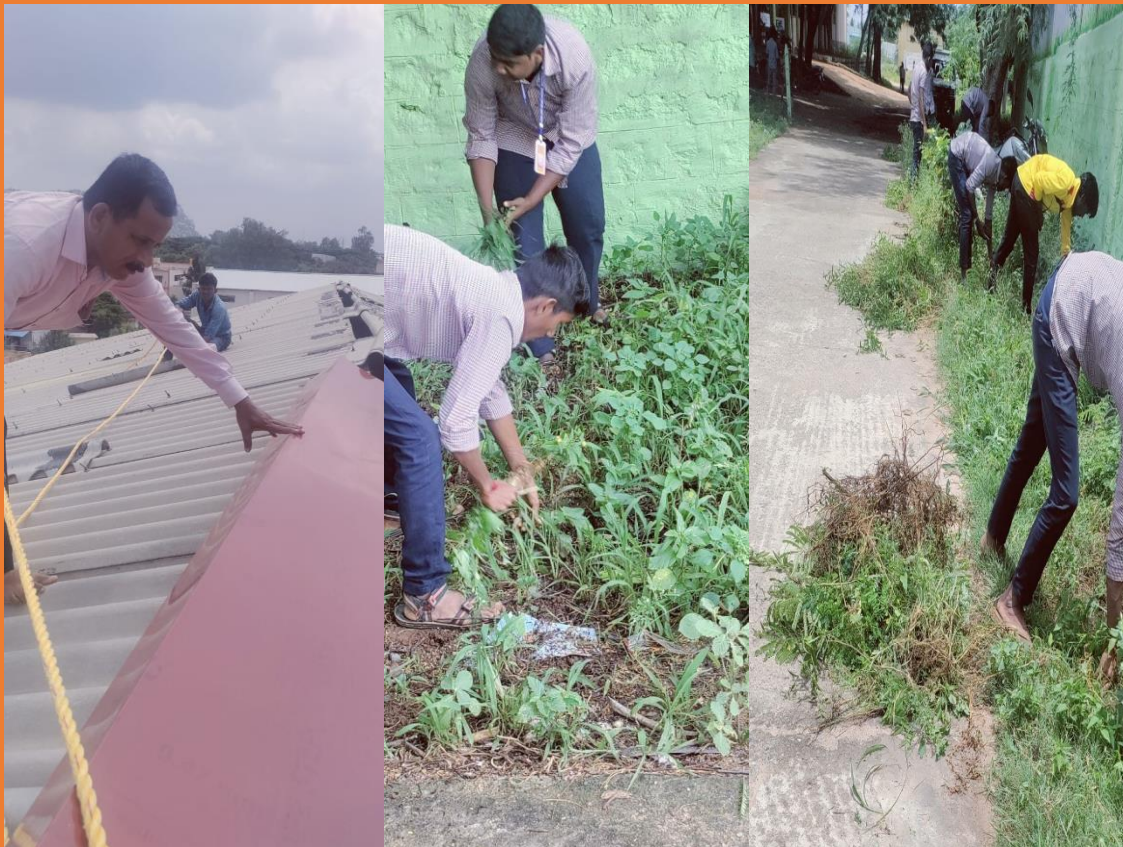
Indoor stadium cleaning and repair activities by our staff member and the students
